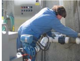
3 – Water treatment plant adjustments
